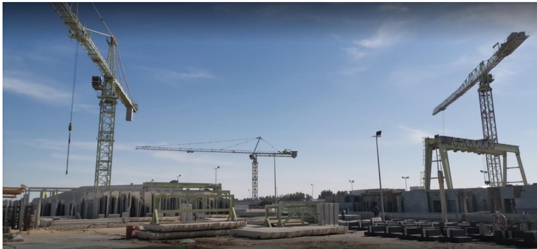
Figure 3.2: Image taken on site showing Saudi Precast Storage Yard with Fixed Cranes and Casting Bed Cranes
