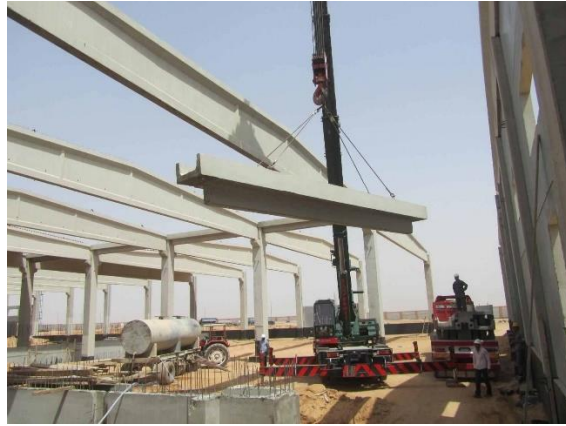
Figure 3.6: Image of rafter beams fixation on site. Drainage raft beam being moved by crane
